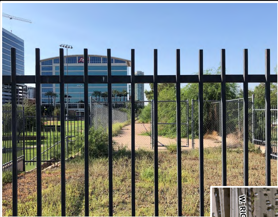
Existing Ash Avenue Roadbed Condition - Looking South towards Rio Salado Parkway
